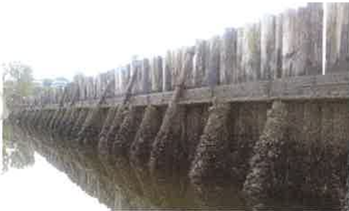
Existing timber pile wall breakwater is severely deteriorated and in need of replacement.
