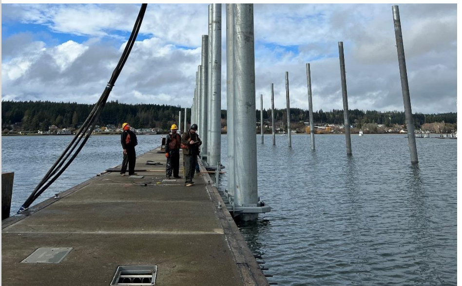
The new floating breakwater is now in place and all piles have been driven to secure it in its final position.
