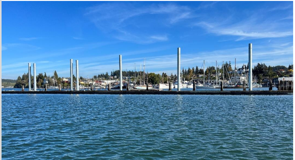
Much of the new west breakwater has already been permanently secured in its final location to replace the protection previously provided by the west log boom. The west log boom is scheduled for demolition in November.
