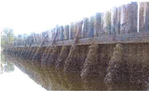
Existing timber pile wall breakwater is severely deteriorated and in need of replacement.
